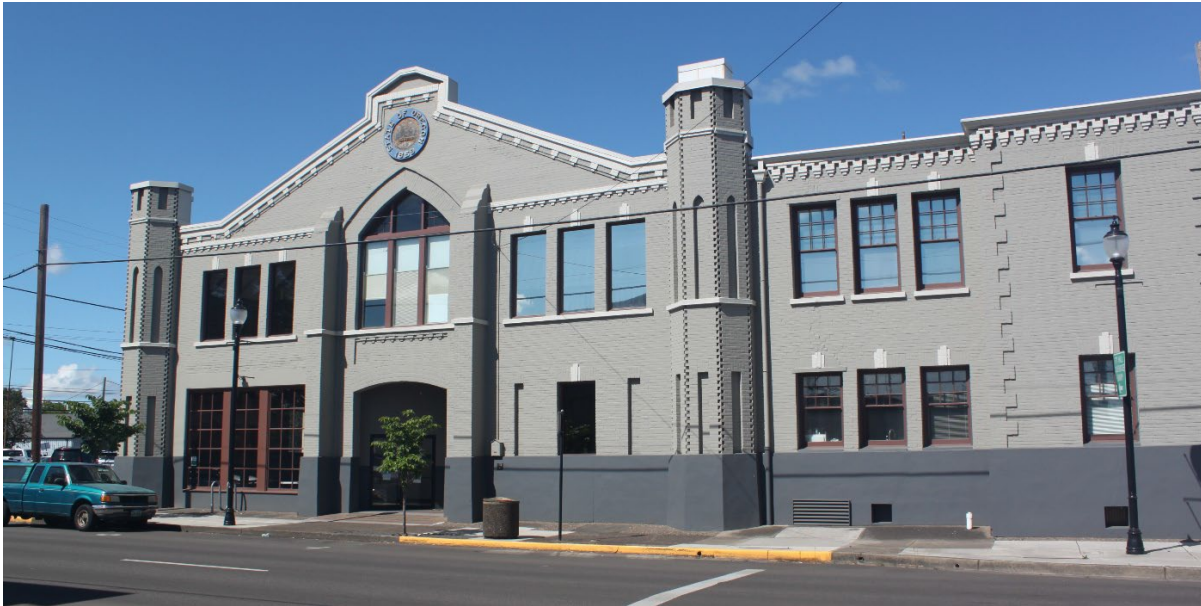
Figure 13. Despite several non-compatible window replacements, the Albany Armory retains most of its character defining features which support its integrity of design, materials, workmanship, feeling and association (AECOM 2021).
